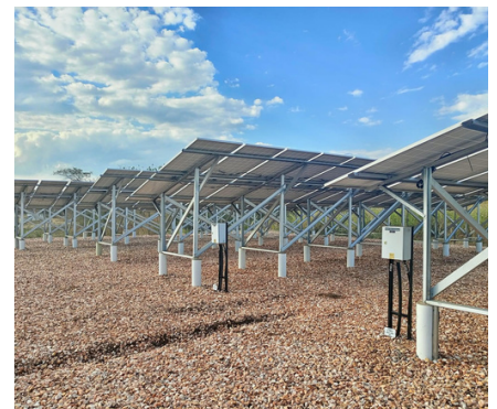
NYIMBA TREATMENT PLANT SOLAR PANELS
