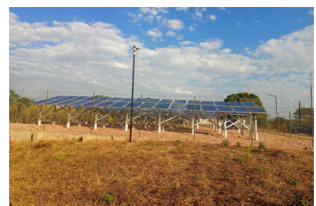
NYIMBA TREATMENT PLANT SOLAR PANELS
